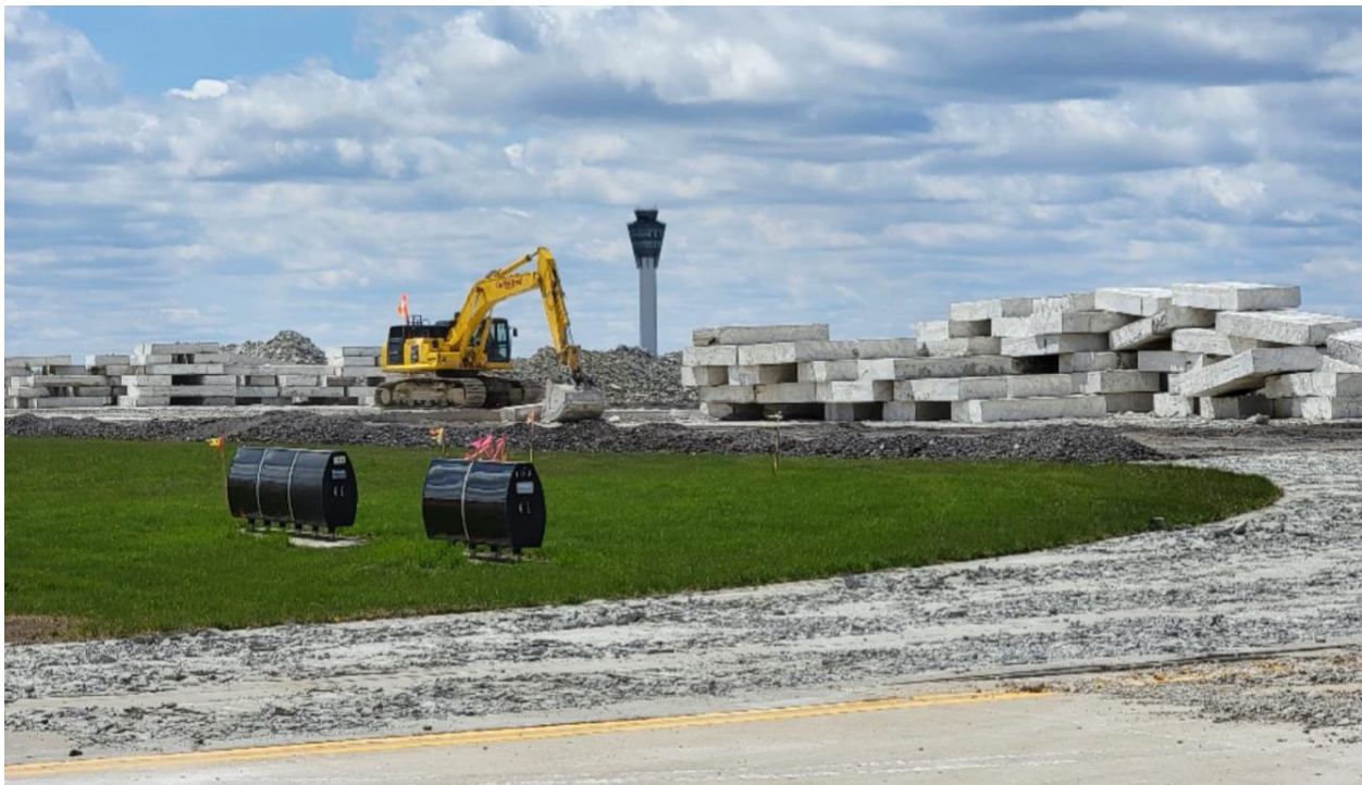
Concrete slabs on the project site at Indianapolis International Airport (photo courtesy Woolpert).
