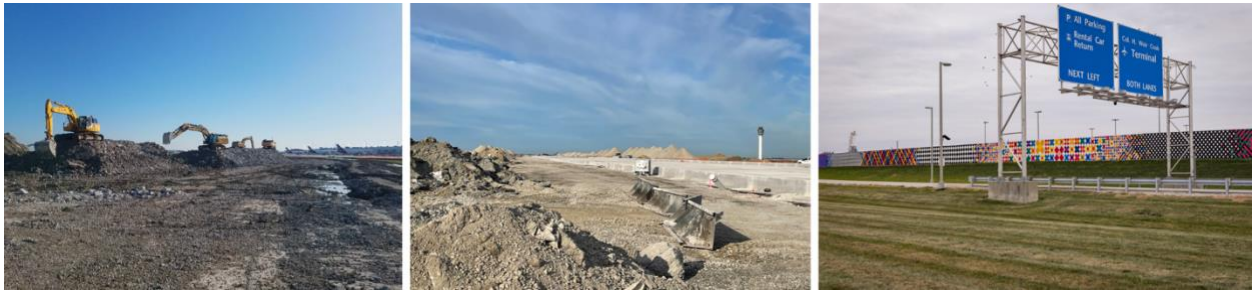
Concrete demo (photo courtesy CTL Engineering); concrete piles (Woolpert); dedication of a three-dimensional mural, “Transitions” (Indianapolis Airport Authority – IAA).
