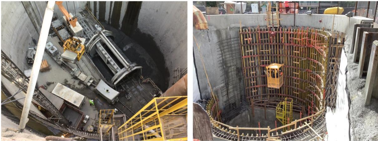
The Ship Canal Water Quality Project includes a 2.7-mile, 18-ft and 10-in internal-diameter tunnel that will extend from Ballard to Wallingford. Left: Ballard Tunnel Segment. Right: Wallingford Shaft Site. December 2022 photos courtesy Seattle Public Utilities.
