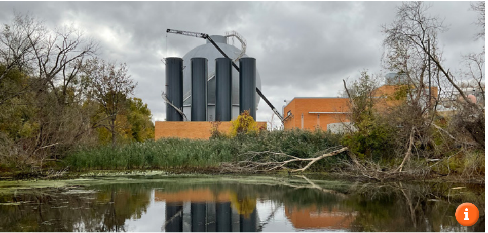
Holland Area Wastewater Reclamation Facility Anaerobic Digester Project, Holland, MI, USA, Envision Gold 2023
