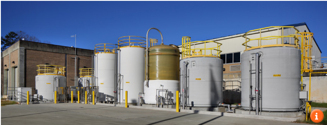
Seneca Water Treatment Plant Improvements, Seneca, SC, USA, Envision Silver 2017
