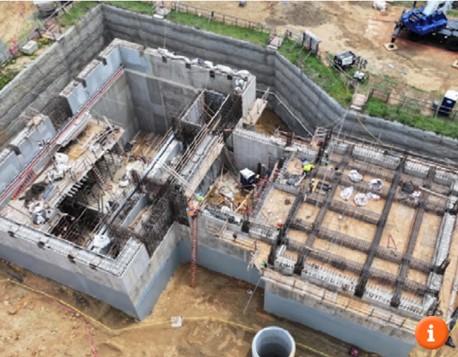
Mallard Creek WRRF Phase 1, Charlotte, NC, USA, Envision Verified 2025
